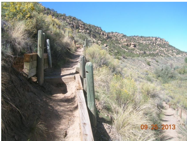
Eroded trail posed safety concerns and side slope stabilization issues.
