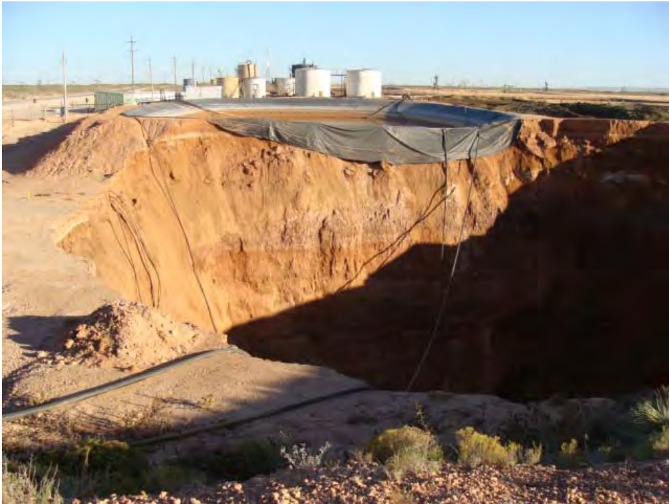
Loco Hills brine well collapse , morning, November 7, 2008, sinkhole with fresh water pond in foreground. Photo courtesy of Oil Conservation Division
