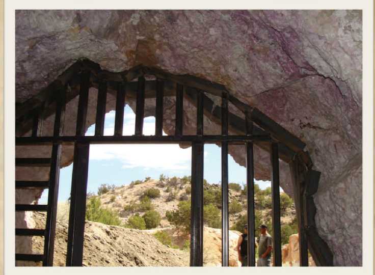
Adit #2 during Construction (July 2011) (Note locking framework against rock profile before grout fill)
