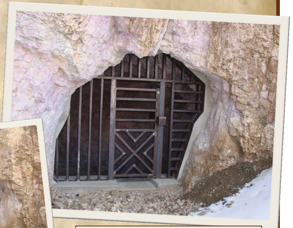
Adit #2 after Construction (Feb. 2012) (Note the pegmatitic crystallization around the mine opening)
