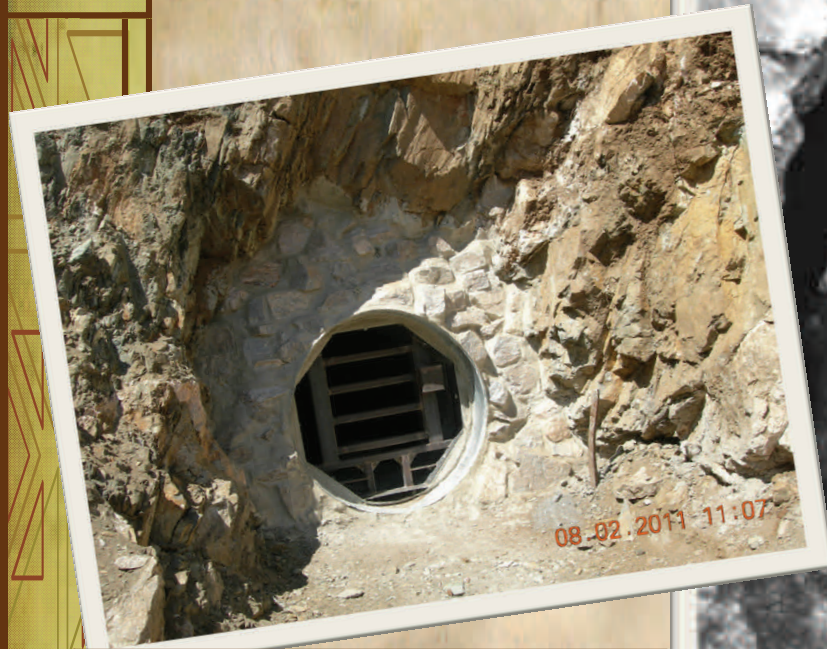
Adit #3 after Construction (Aug. 2011) (Note bat compatible and small mammal access openings)
