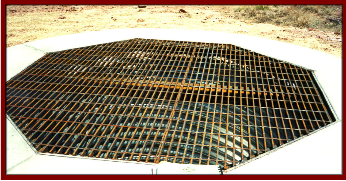
Close-up of the grated closure at the Feature 11 Shaft, showing the corrugated steel pipe riser (inside a polyurethane foam plug and masonry collar)
