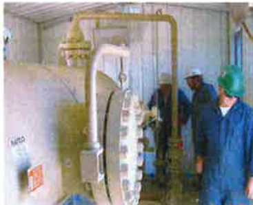
Portable Three Phase Separator, Source: BP
