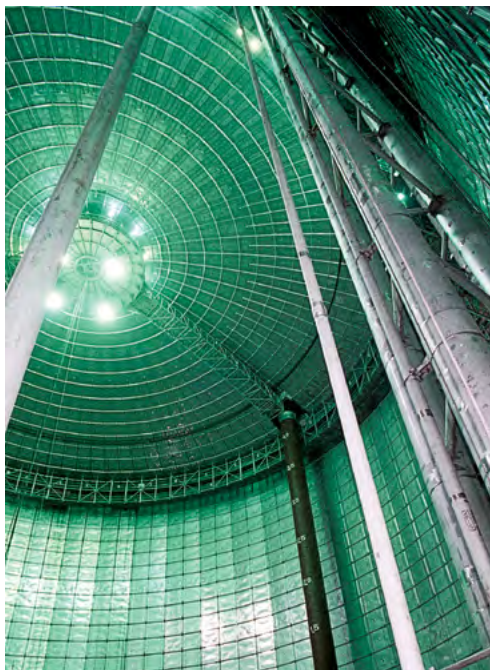
Picture 7.4: Still-pipe cluster inside an LNG tank.
