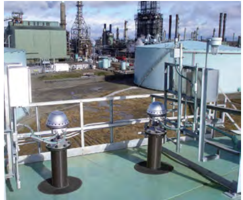
Figure 9.3: Tank redundancy is accomplished with dual tank gauges and separated communication layers - wired and wireless.
