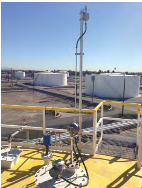
Figure 9.8: Antenna connected to tank devices.
