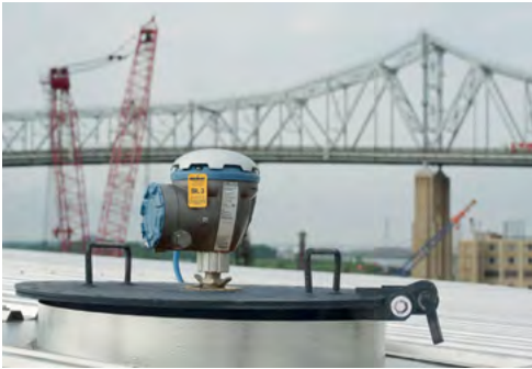
Figure 2.10: Modern radar level gauge on a fixed roof tank.
