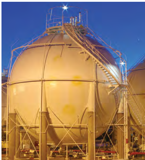
Figure 3.5: Level measurement in pressurized tanks cannot be done by hand gauging, leading to technology specific recommendations for servo based and radar based level gauging.
