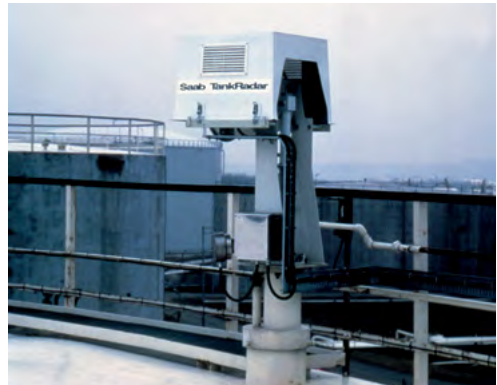
Figure 2.9: First high precision radar gauge installed in 1985 on a refinery tank.
