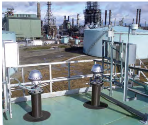
Figure 9.3: Tank redundancy is accomplished with dual tank gauges and separated communication layers - wired and wireless.
