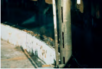
Figure 2.16: Low loss mode radar measurement can be used to virtually eliminate measurement degradation in old still-pipes.
