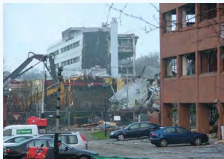
Figure 10.1: Property damage after the accident at Buncefield.
