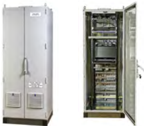
Figure 9.5: A tank gauging system cabinet.
