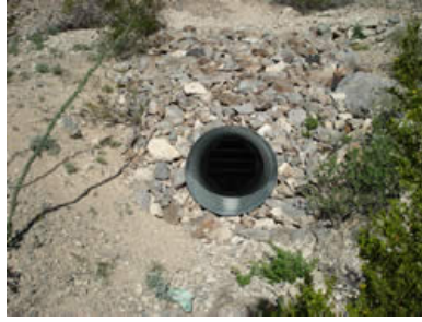
A culvert with a bat gate has been constructed at the adit entrance.
