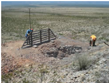
A unique bat gate constructed at the entrance to the shaft. High tensile steel mesh was attached to the gate and covered the shaft. Barn owls continue to use the gate for entry.
