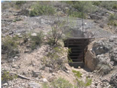
Bat gate constructed at the entrance to the adit. High tensile steel mesh was installed above the gate along with a raptor perch.
