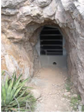
A bat gate built at the adit entrance.
