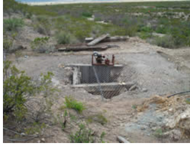
High tensile steel mesh now cover the shaft opening. Potential access to water is preserved.
