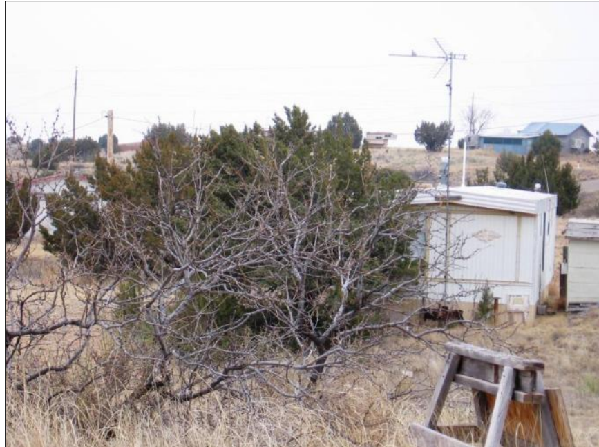
Figure 5.3. Structure requiring defensible space and fuels mitigation.
